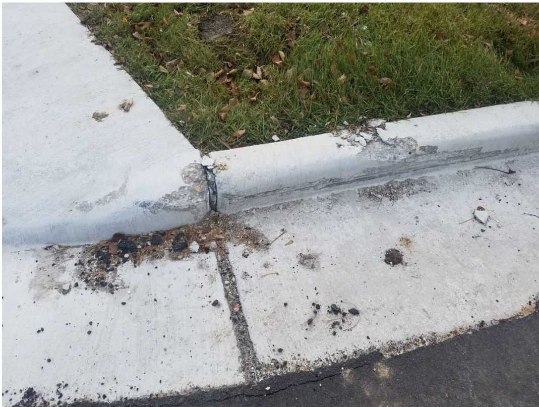
Curb Damage – Winter 2019/2020
