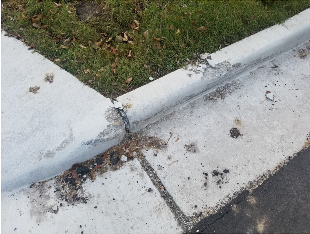
Curb Damage – Winter 2019/2020
