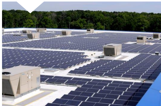
Commercial Solar Array, Photo from Milwaukee Journal Sentinel
