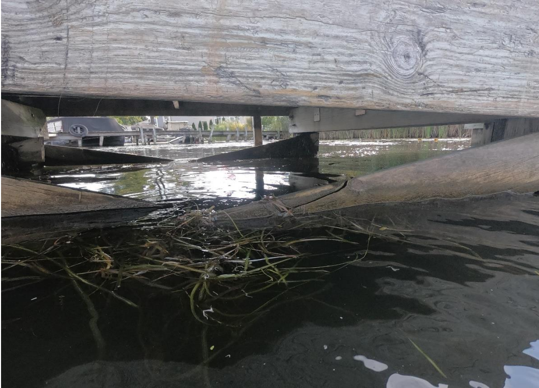
NW Corner of East pier with split cross brace on west edge.
