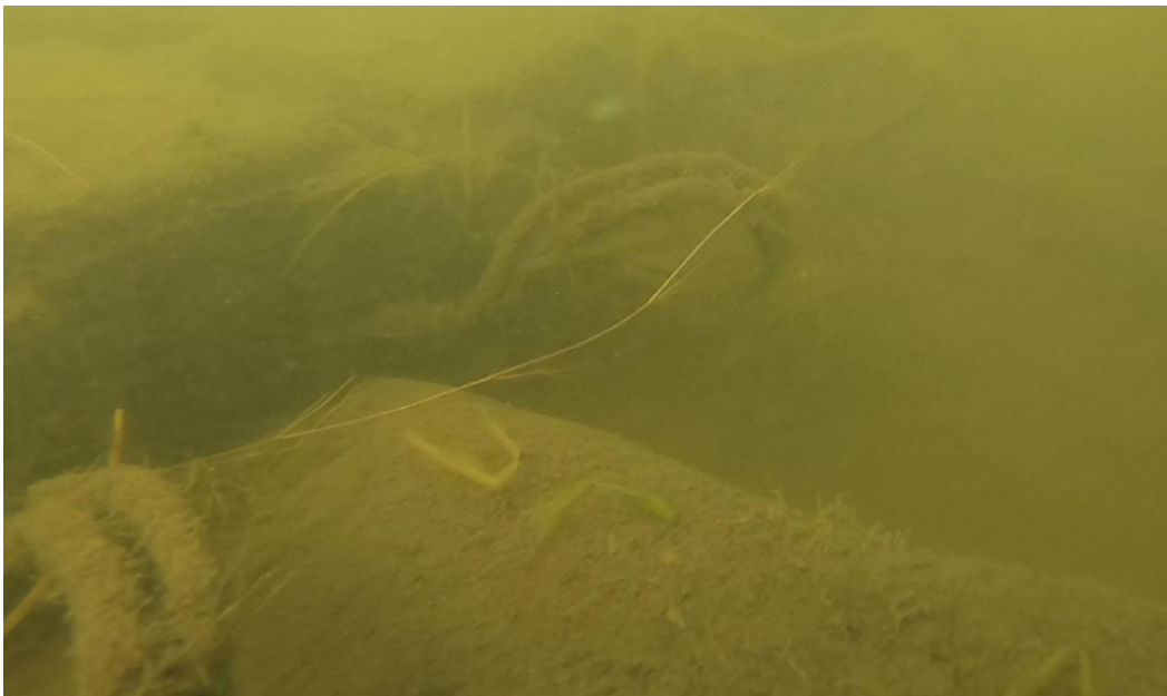
Typical view of the end of revetment mat (cable loops visible) with exposed geotextile fabric.
