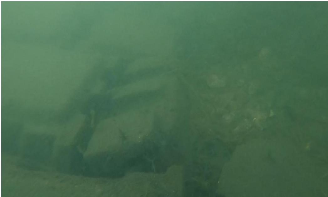
Displaced/Misaligned blocks - Blocks are seen embedded on side, missing and misaligned in photo.
