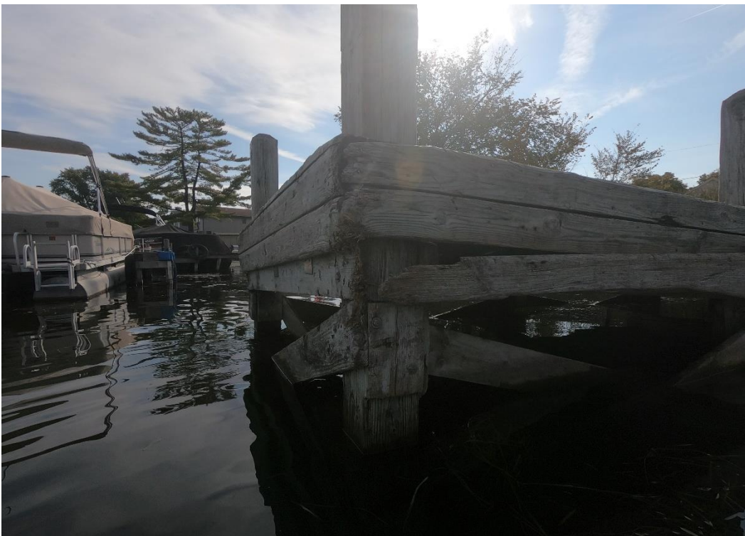
NW Corner of East pier with impact damage.
