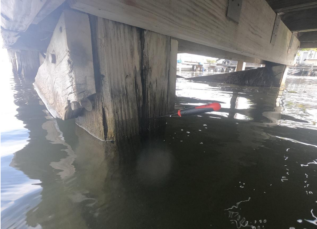
East pier column with surface check and minor deterioration. Damaged cross brace also shown.
