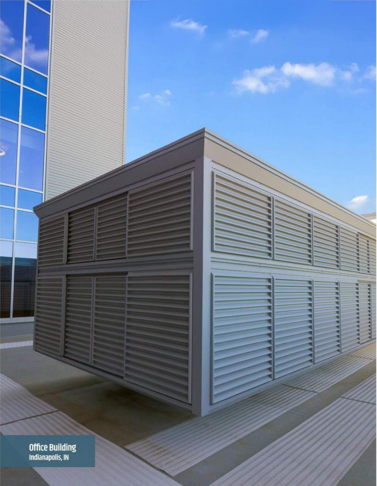
ROOF TOP EQUIPMENT SCREENS
