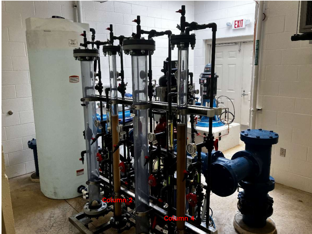
Figure 5. PFAS Pilot System
