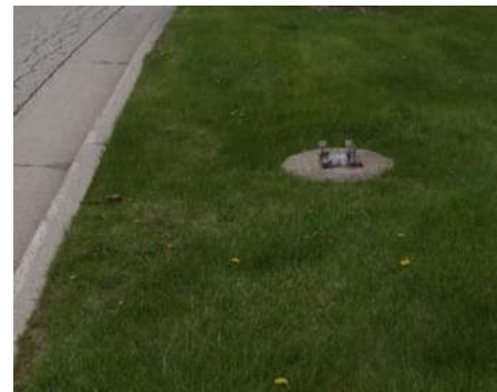
Abandoned light pole base
